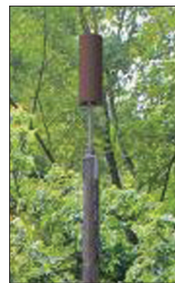
A cellphone antenna
